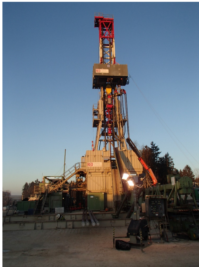
Figure 1: Running casing using the RED E-200 rig at the Anshof-3 drill site
